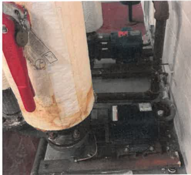
Figure 9: Hot Water Pump (P-3, and P-4)
