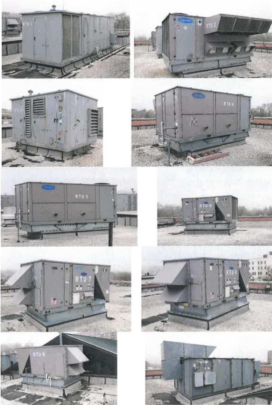
Figure 6: RTU-1 to RTU-9, and AHU-1
