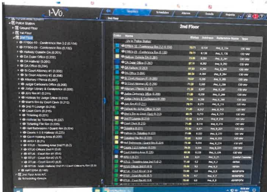
Figure 17: Typical Space Temp Overview Screen
