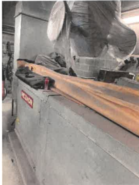
Figure 7: AHU-1 at Basement (Reznor air handler with only heating coil)
