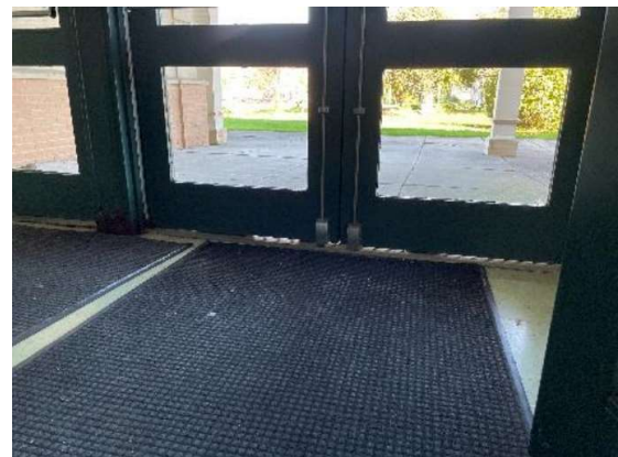
Entry Door Gap
