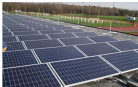
Recent Siemens Installation
