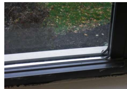
Failed Gasket on Window
