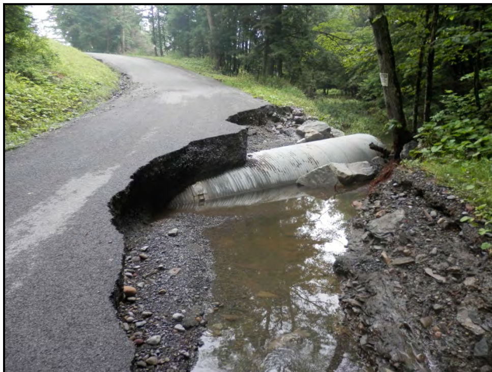
Damage to Abbert Road in the Town of Madison (Source: Madison County)
