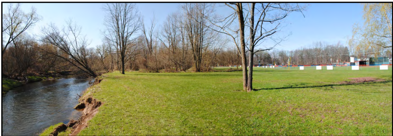
Streambank erosion adjacent to Maxwell Field
