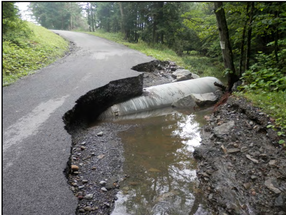
Damage to Abbert Road in the Town of Madison (Source: Madison County)
