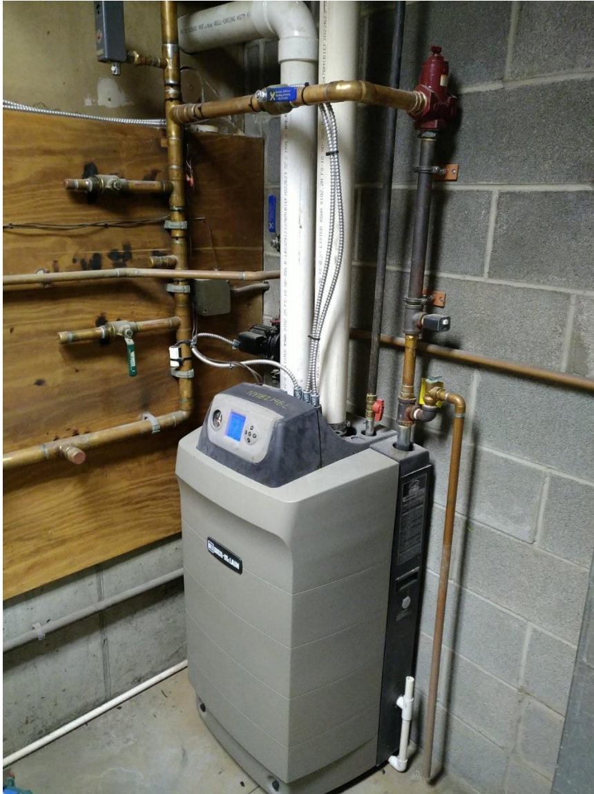
Photo: The Town Barn water heater uses this boiler to heat the water.
