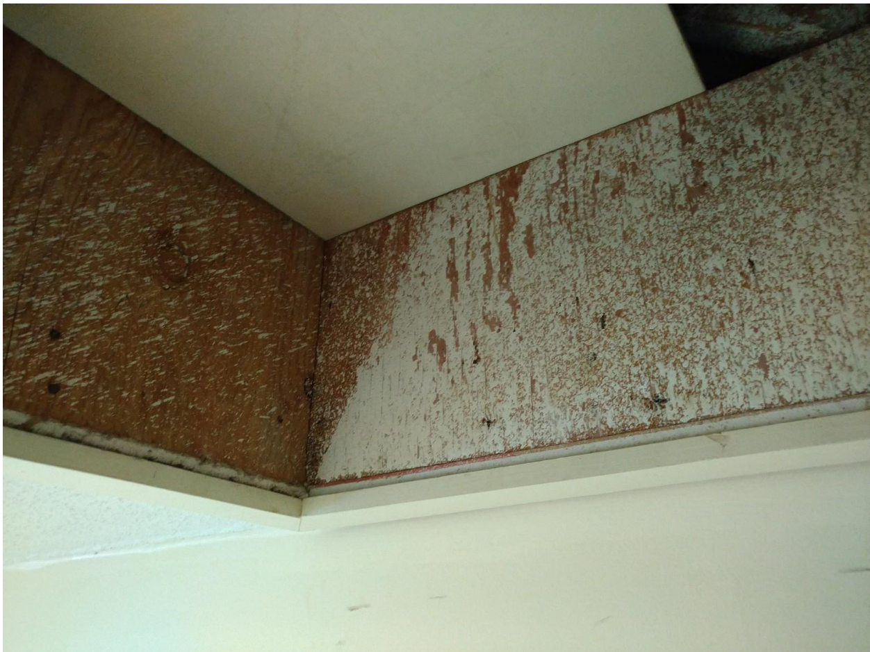
Photo: This attic hatch has no weather-stripping or insulation.
