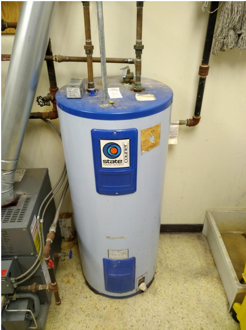
Photo: The Town Hall water heater is a very old electric resistance tank-style heater.
