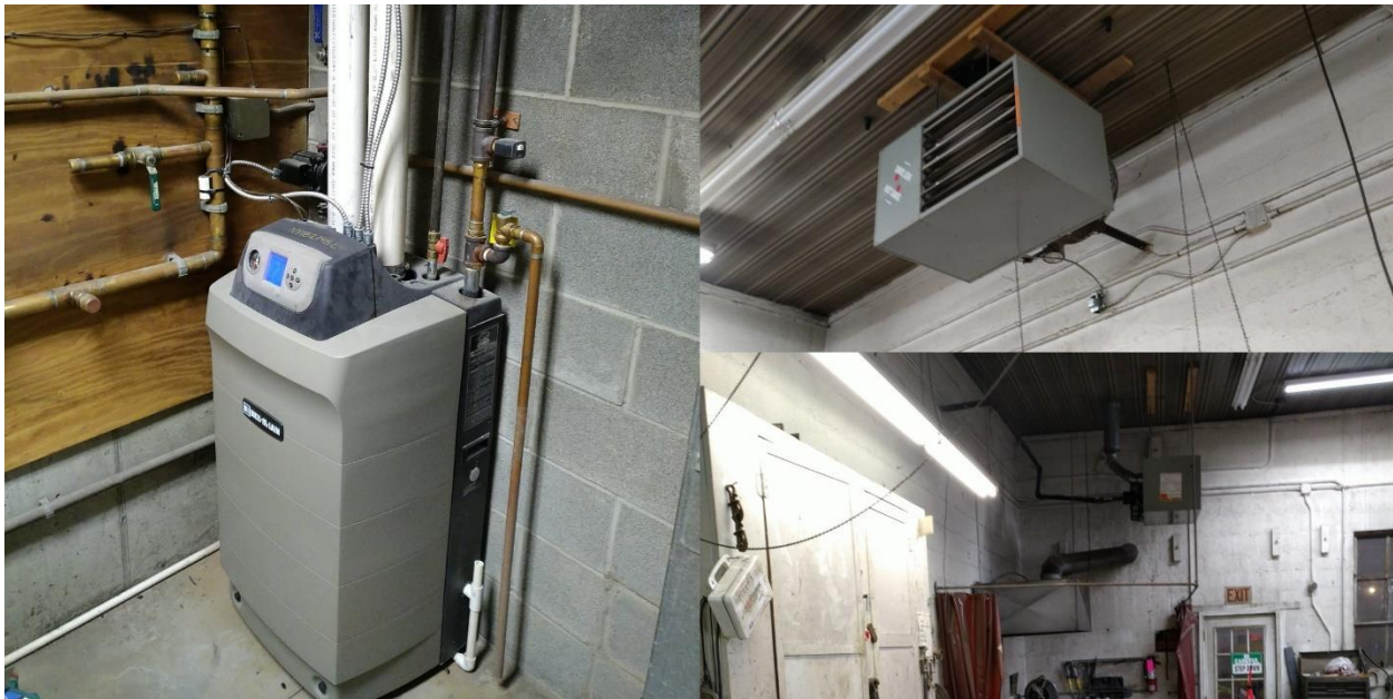
Photo: The Town Barn is heated by a gas fired boiler and two gas fired unit heaters.
