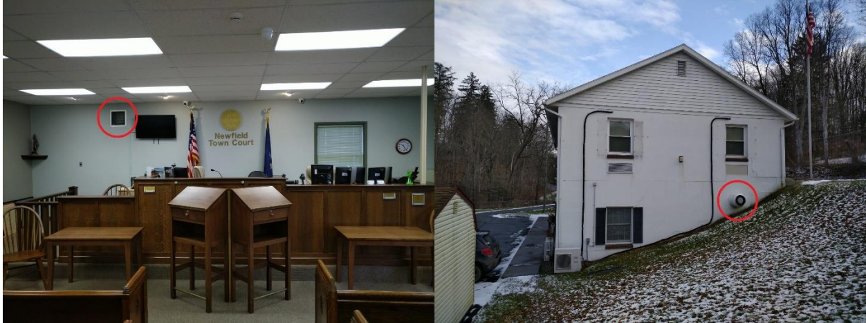
Photo: This exhaust fan serves no purpose currently and allows for significant air leakage.
