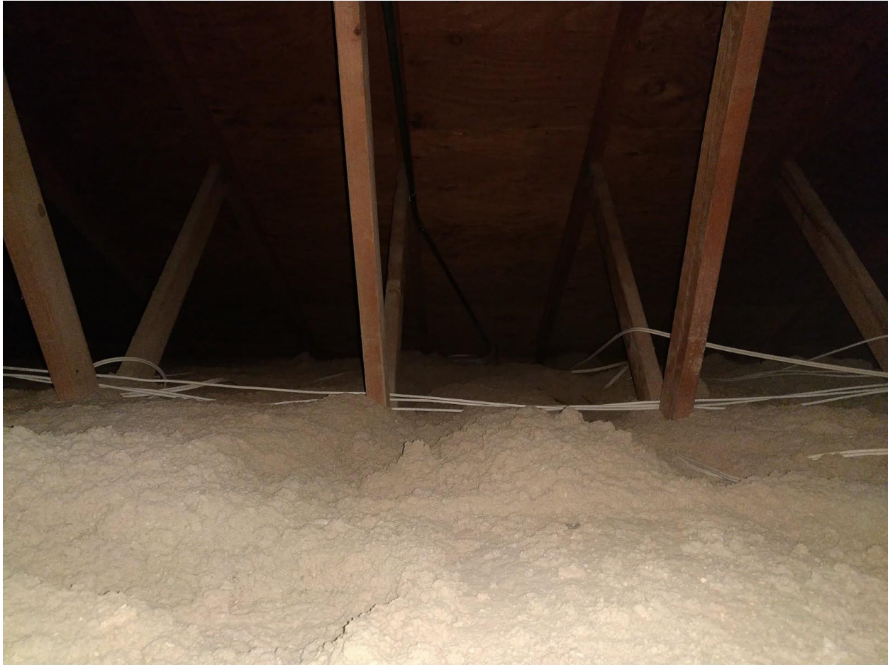
Photo: The insulation is evenly distributed and appears to be in good condition.
