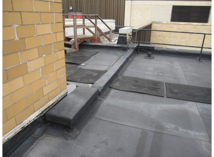
Figure D.6: Building 3—Detail view of curbs at west edge of roof
