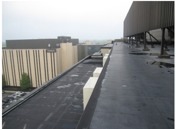
Figure D.11: Building 16—Overall view of roof showing typical roof edge, looking north
