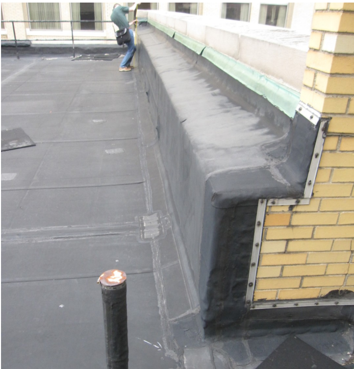
Figure D.3: Building 3—Detail view of existing parapet at east roof edge
