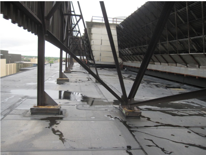
Figure D.10: Building 16—Overall view of roof including cooling towers, looking north
