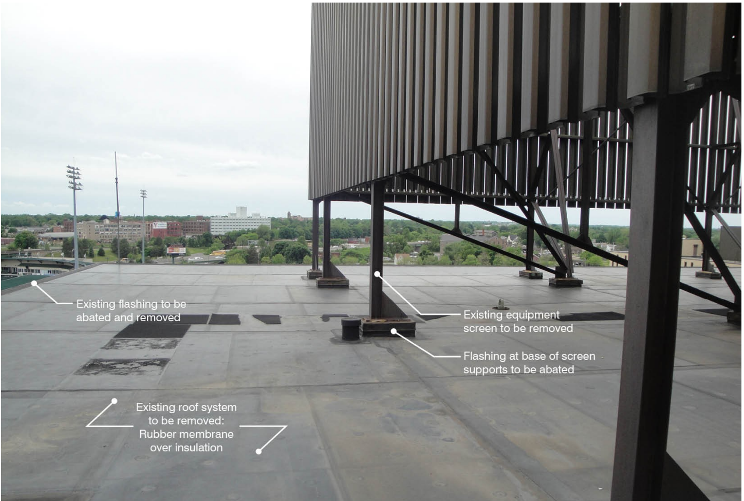
Figure D.19: Building 16. View of existing roof, looking south west. Notes indicate proposed demolition work necessary for installation of vegetated roof system.
