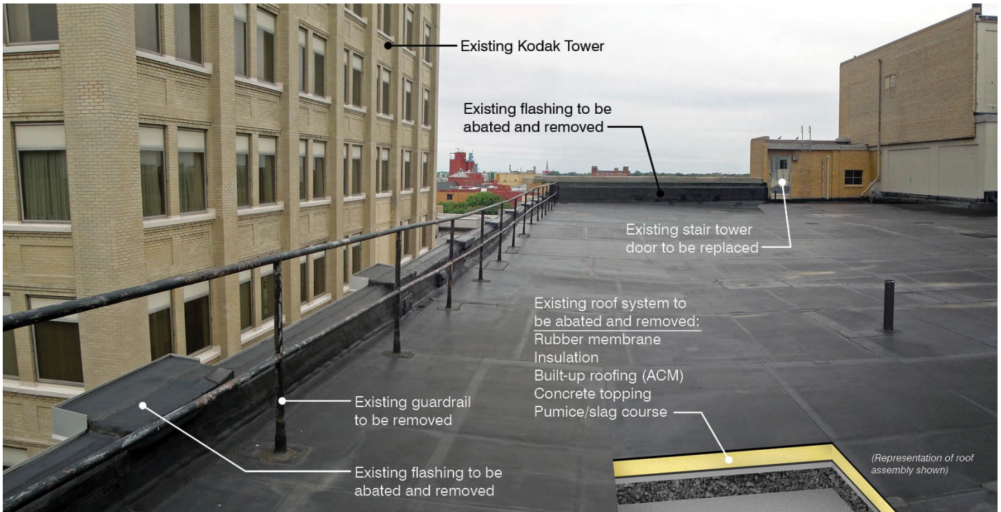
Figure D.17: Building 3. View of existing roof, looking north east. Notes indicate proposed demolition work necessary for installation of vegetated roof system.
