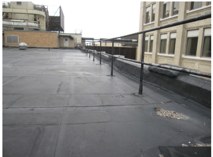
Figure D.4: Building 3—Detail view of existing guardrail at north roof edge
