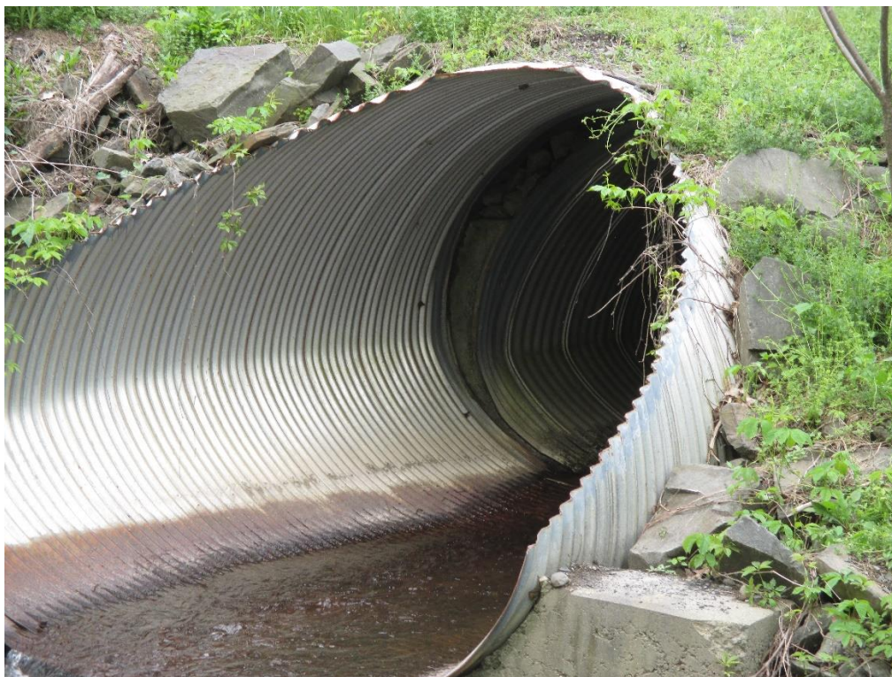
Photo 2: Disconnected outlet end piece – looking southwest.
