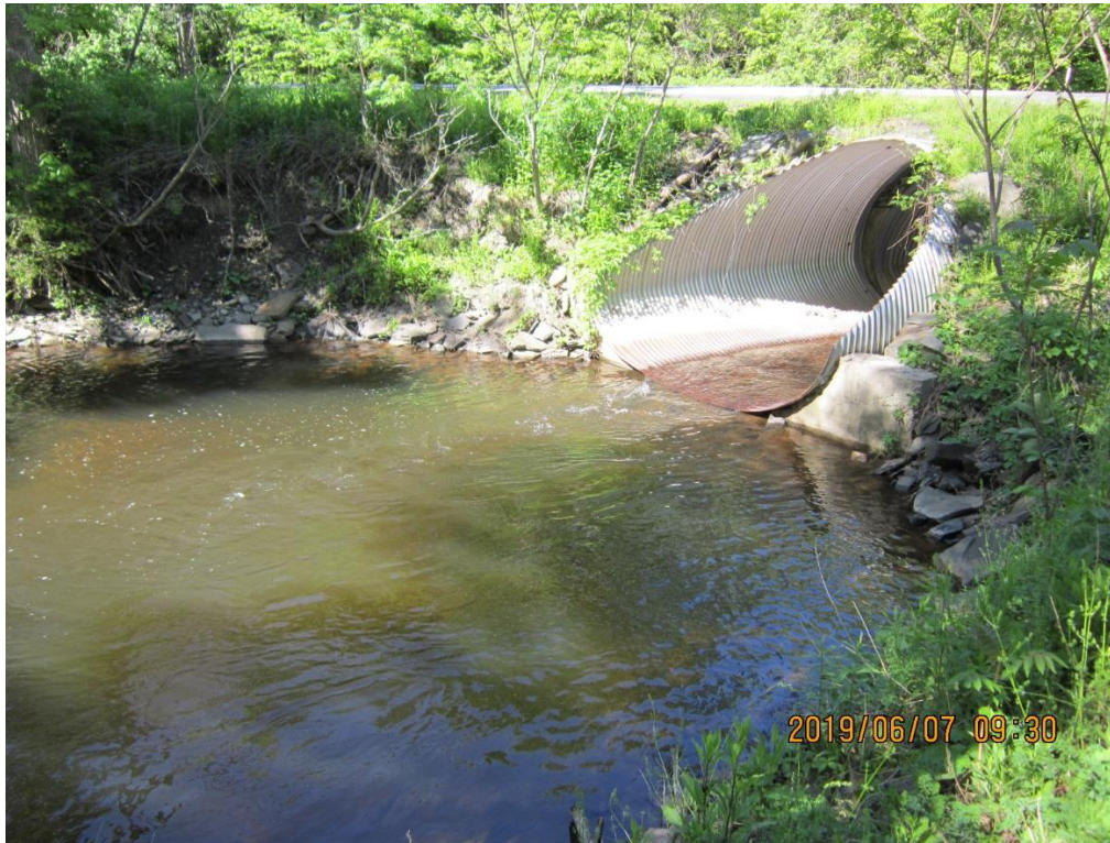
Photo 1: View looking southwest at east side (outlet) of Culvert. County Route 6 above.
