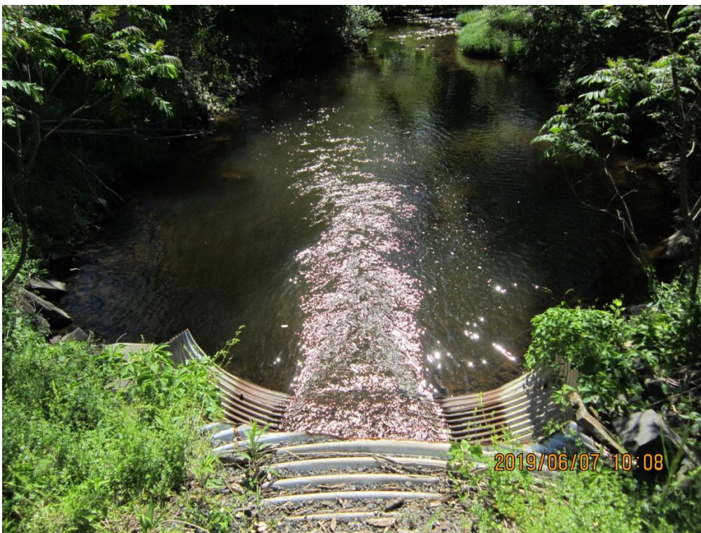
Photo 4: View looking east at outlet of Culvert and downstream – from edge of highway.
