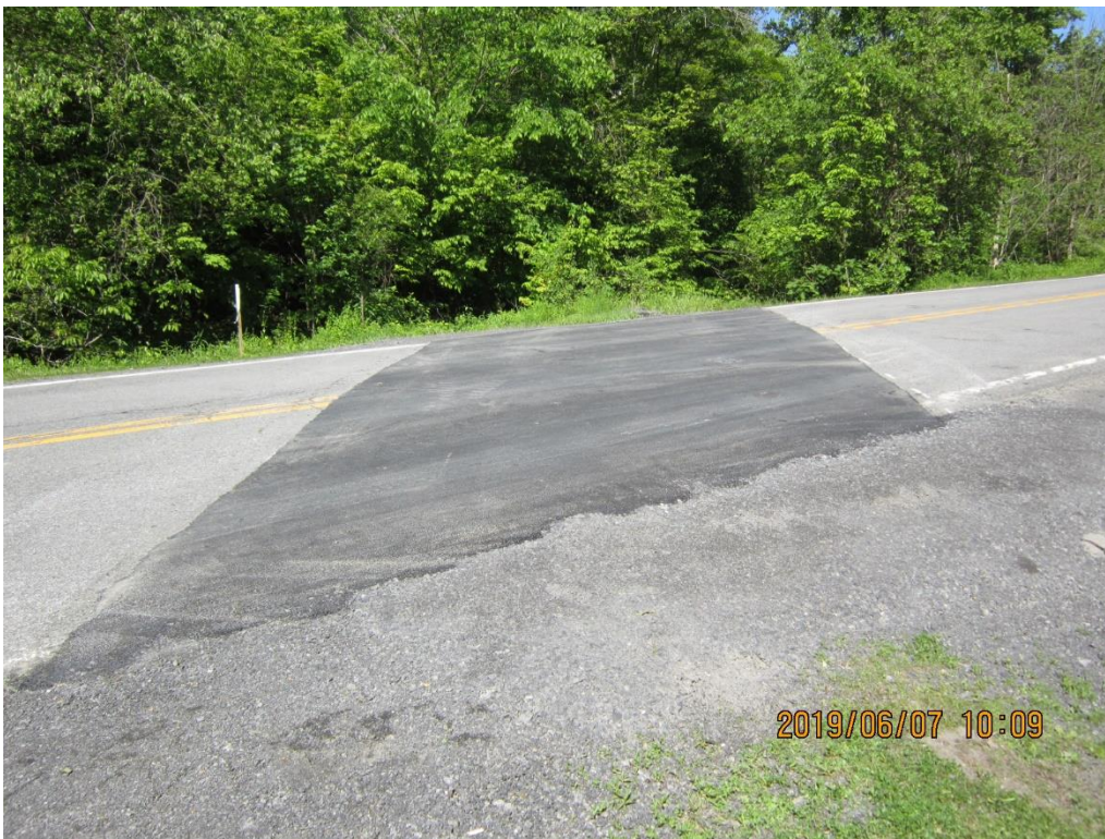
Photo 10: Asphalt patch over Culvert – looking northwest.
