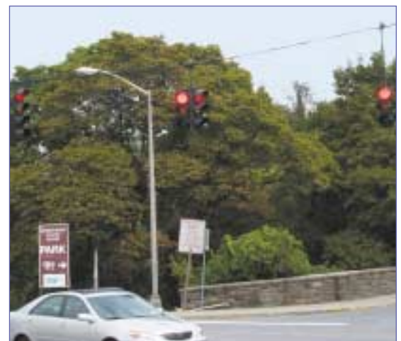
An installation of red LED signals in the Westchester County service area.
