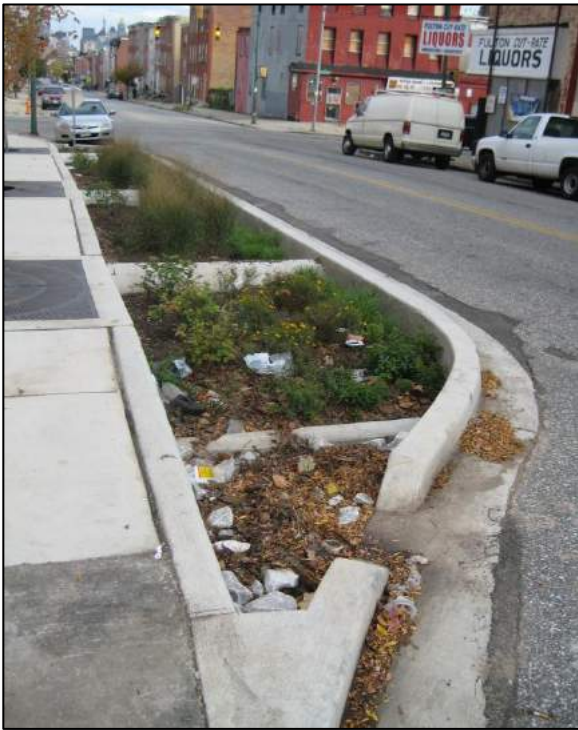
The above picture depicts a curb extension which allows for the inflow of storm water runoff.
