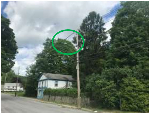
Mill St., Dover Plains street lights after upgrade
