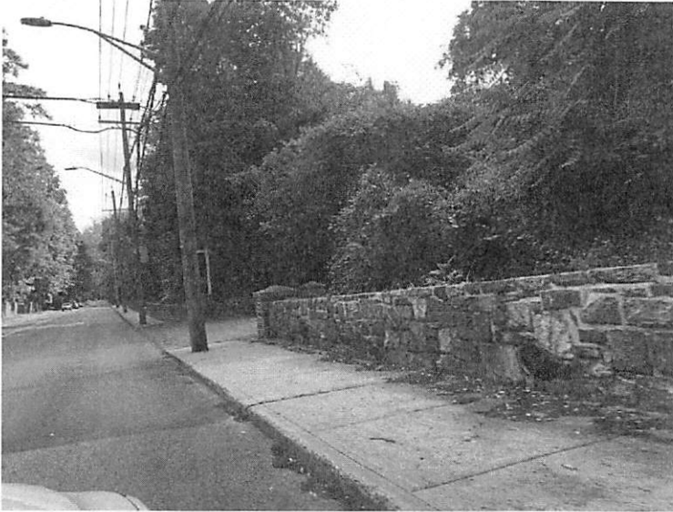
Figure 20 Example of a row of utility poles that Violates the ADA Minimum Sidewalk Width Requirement
