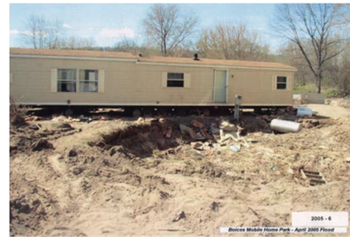
2005 - 6 Flood Damage in Boice's Mobile Home Park, Farm to Market Road, Town of Ulster, April 2005.
