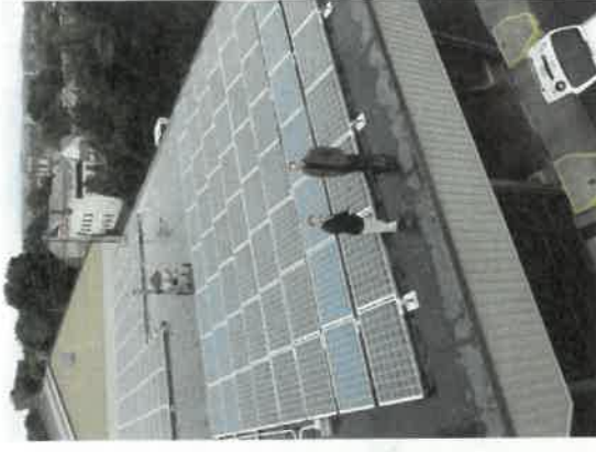
City of Watervliet Solar Installation
