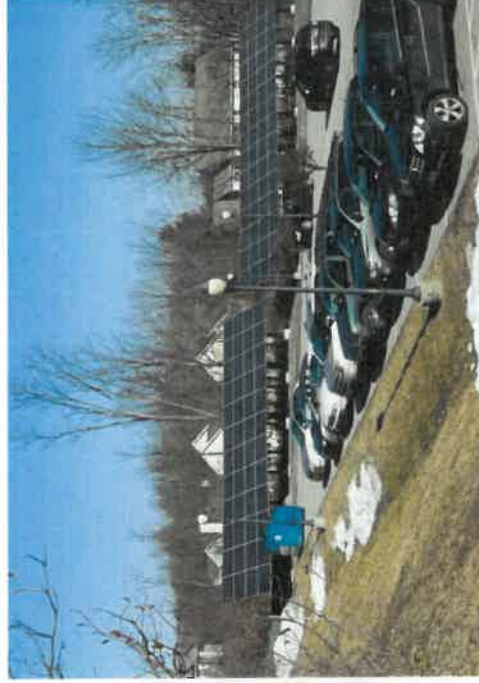
Town of Niskayuna Solar Installation
