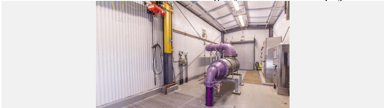
Purple pipes inside Riverhead’s Advanced Wastewater Treatment Facility carry re-usable water for irrigation.
