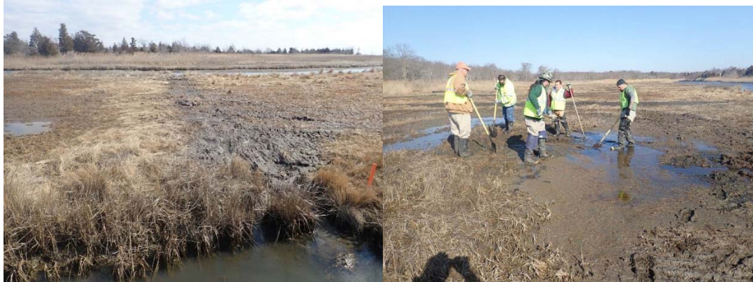
Left: A finished ditch with coir logs covered with sediment. Right: Runnels being hand dug. These runnels help prevent stagnant water, preventing mosquito breeding
