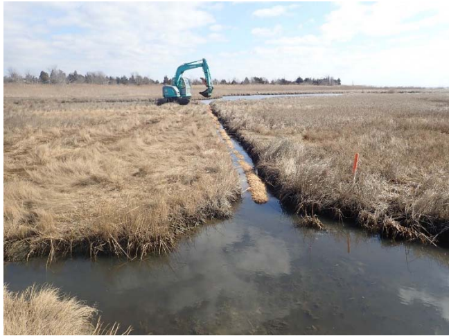
Coir logs placed in a ditch prior to having sediment placed on top of them.
