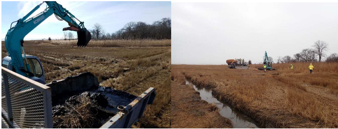
Left: Tidal channels are being cleaned here, and the material being pulled out will be used to fill in ditches. Right: Coir logs being brought out to the marsh on the Rotary Ditcher with help from the Kobelco Excavator.
