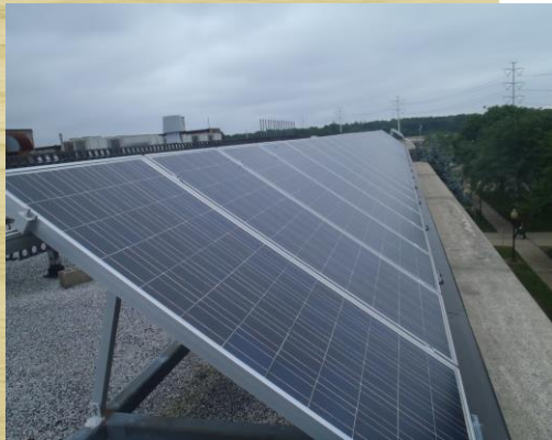
46.6 kW array of Solar Panels
