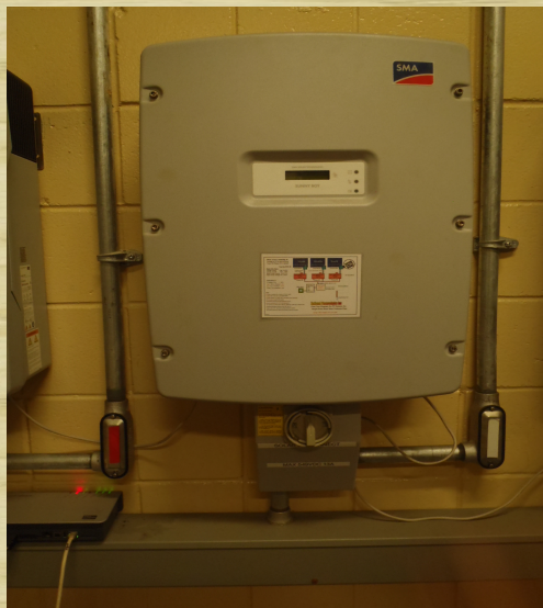
Disconnect Box for the Solar Panels on the roof
