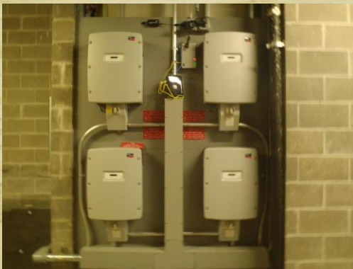
Solar Inverters that change solar energy to electrical
