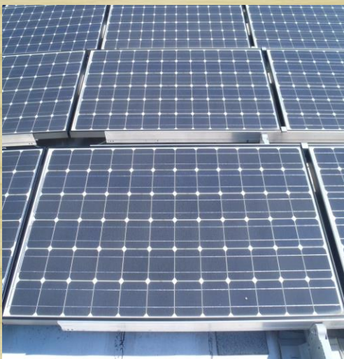
Close up on the Solar Panel array configuration
