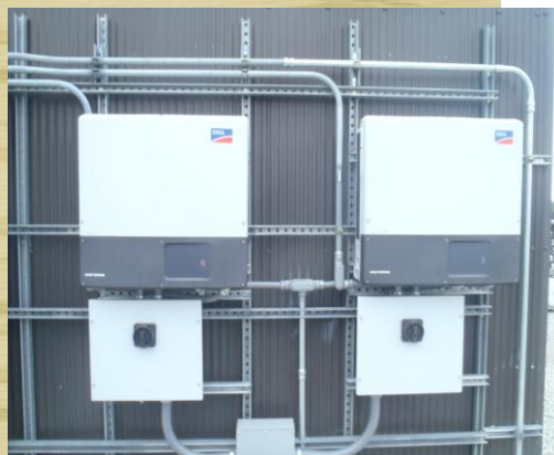
Two disconnect boxes that control the Solar Array
