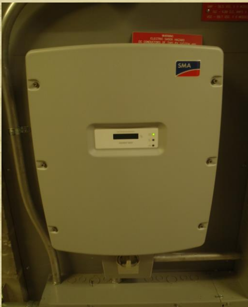
Singular Solar Inverter
