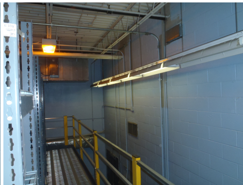
Shown above are the lighting in the Ready Room (Mezzanine Level)
