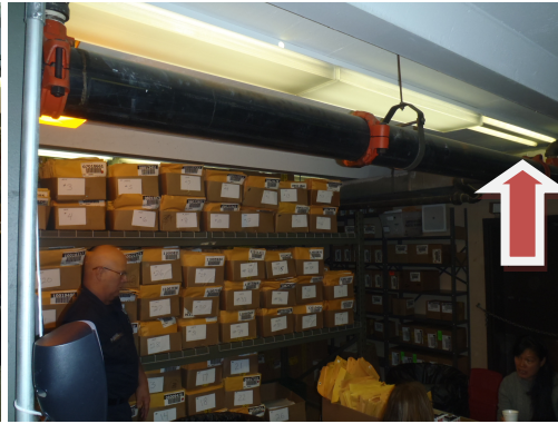
Shown above are the light fixtures in the vault area with missing lens
