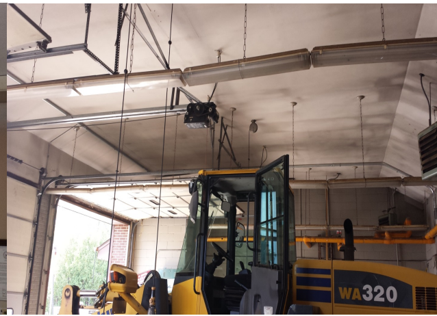
Shown above is lighting in workshop
