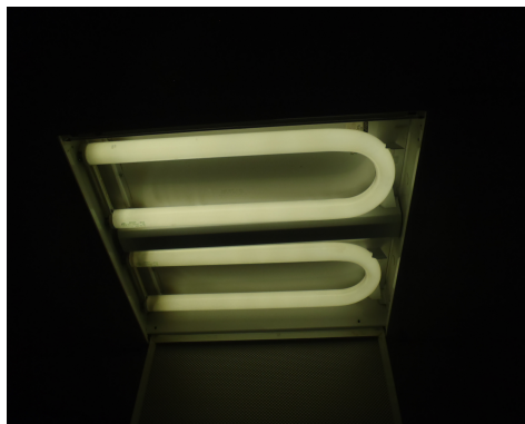
Shown above is a 2 x 2 U-tube fixture with missing lens.
