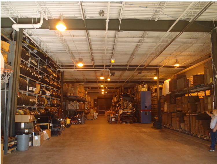
Shown above is general lighting in the warehouse area
