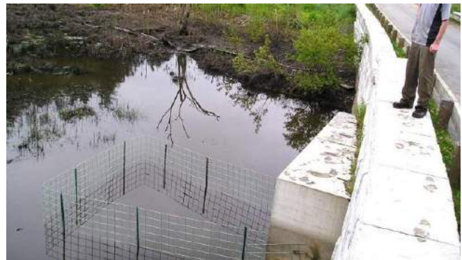
Culvert fences are the most commonly used beaver device by the Forest Service, however they may block fish passage. USFS concludes that the best solution is culvert replacement. Source: www.beaversolutions.com
