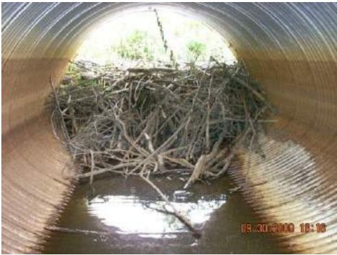
Undersized culverts, which constrict flow, are almost irresistible to beavers. Source: www.martinezbeavers.org/wordpress
