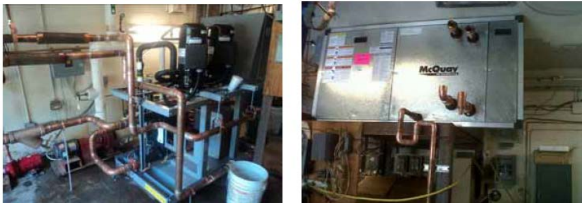
* New Carrier Chiller on left and New McQuay AHU on right at DPW Building*
