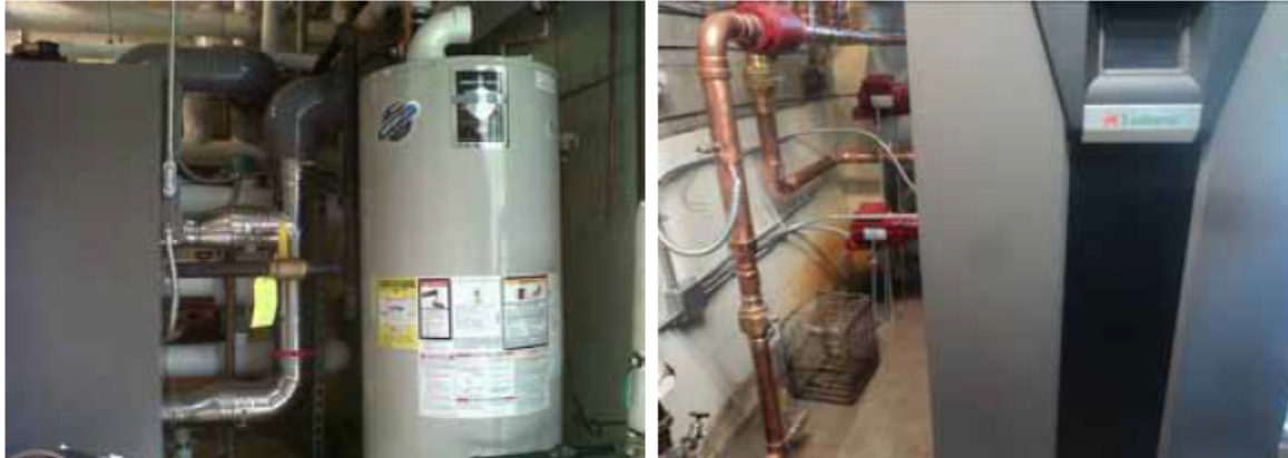
* New DHW Heater (Left) Lochinvar Boiler at DPW Building (Right)*
