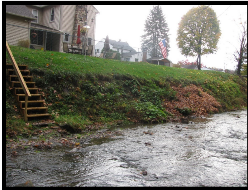
Looking East at Erosion Hazard at a Private Home.
