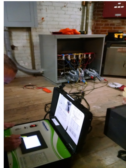
Figure 14 – Transformer Loss Test
