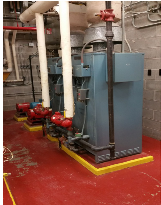
Figure 11 –Jail Boilers (Precision)
