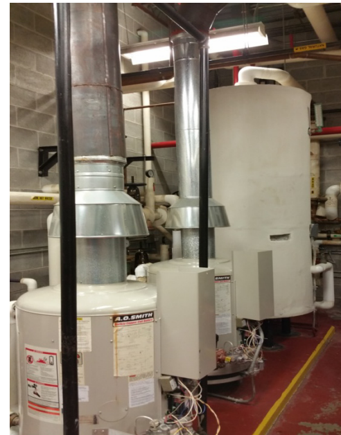
Figure 12 – Jail Domestic Hot Water System
